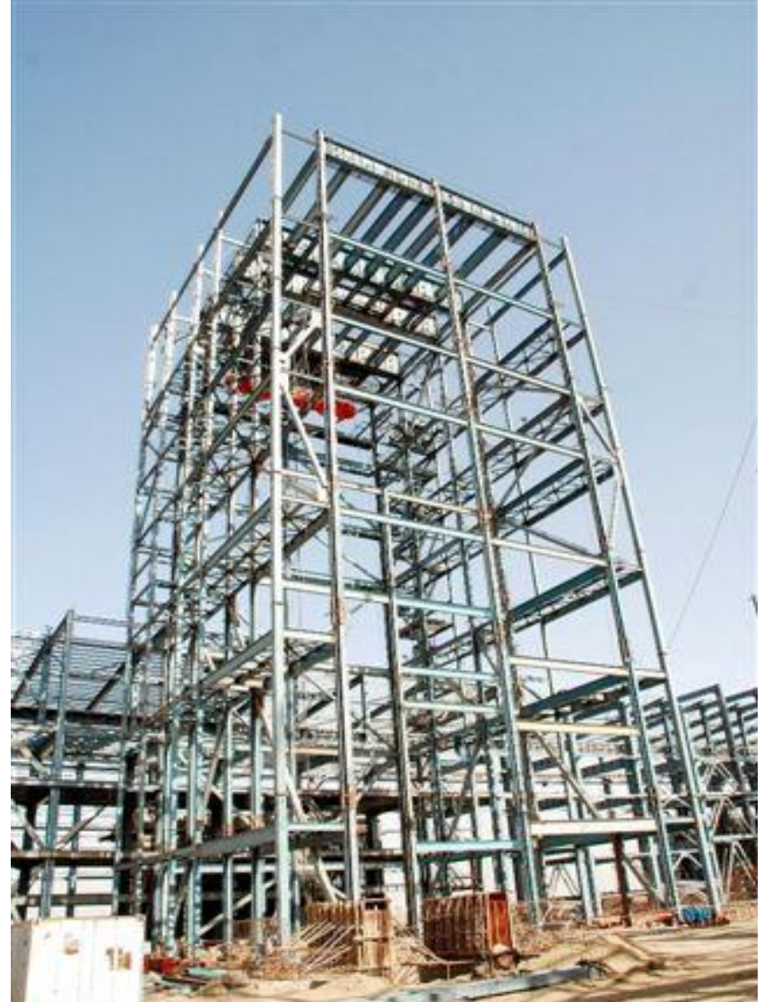
Boiler Structure 1 with drum
