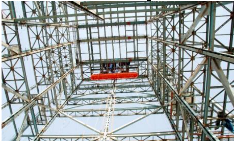
Boiler Structure 1 with drum
