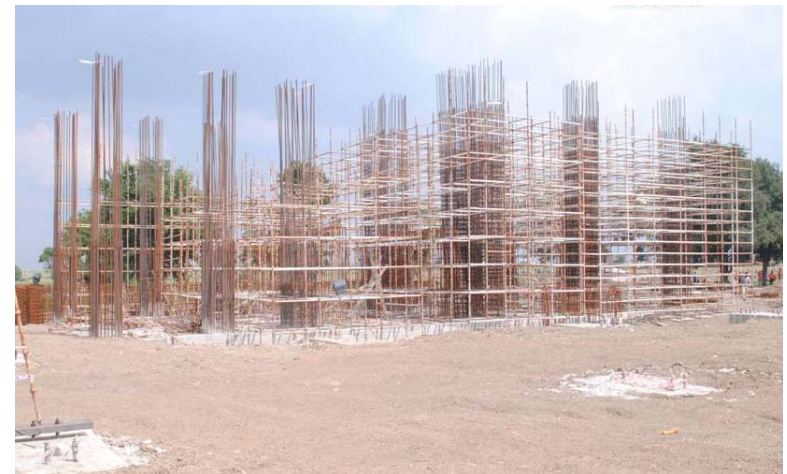
Turbine Generator Deck
